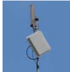
A typical Village Networks node aerial, which distributes the broadband connection to several locations.
