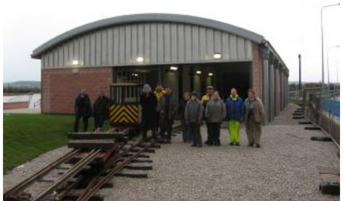
The track-laying gang on 4 th March included visiting volunteers from the Sherwood Forest Railway in Nottinghamshire. Thanks to their help most of the new tracks are already nearly finished.
