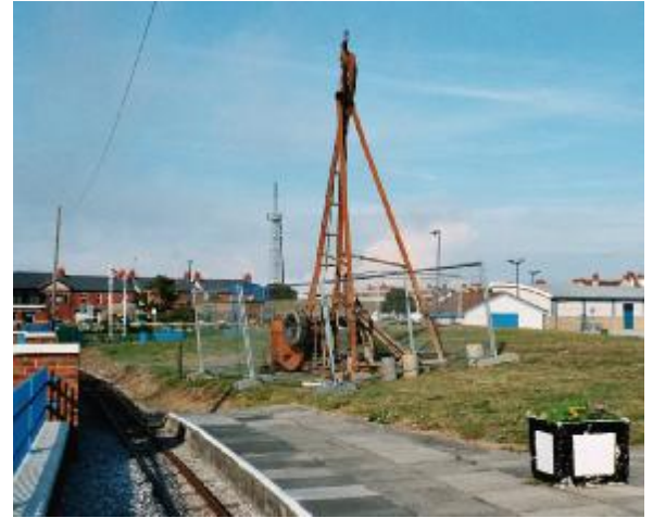
Drilling in progress to establish ground conditions, on 11 th July. This work alone cost £6,000.
