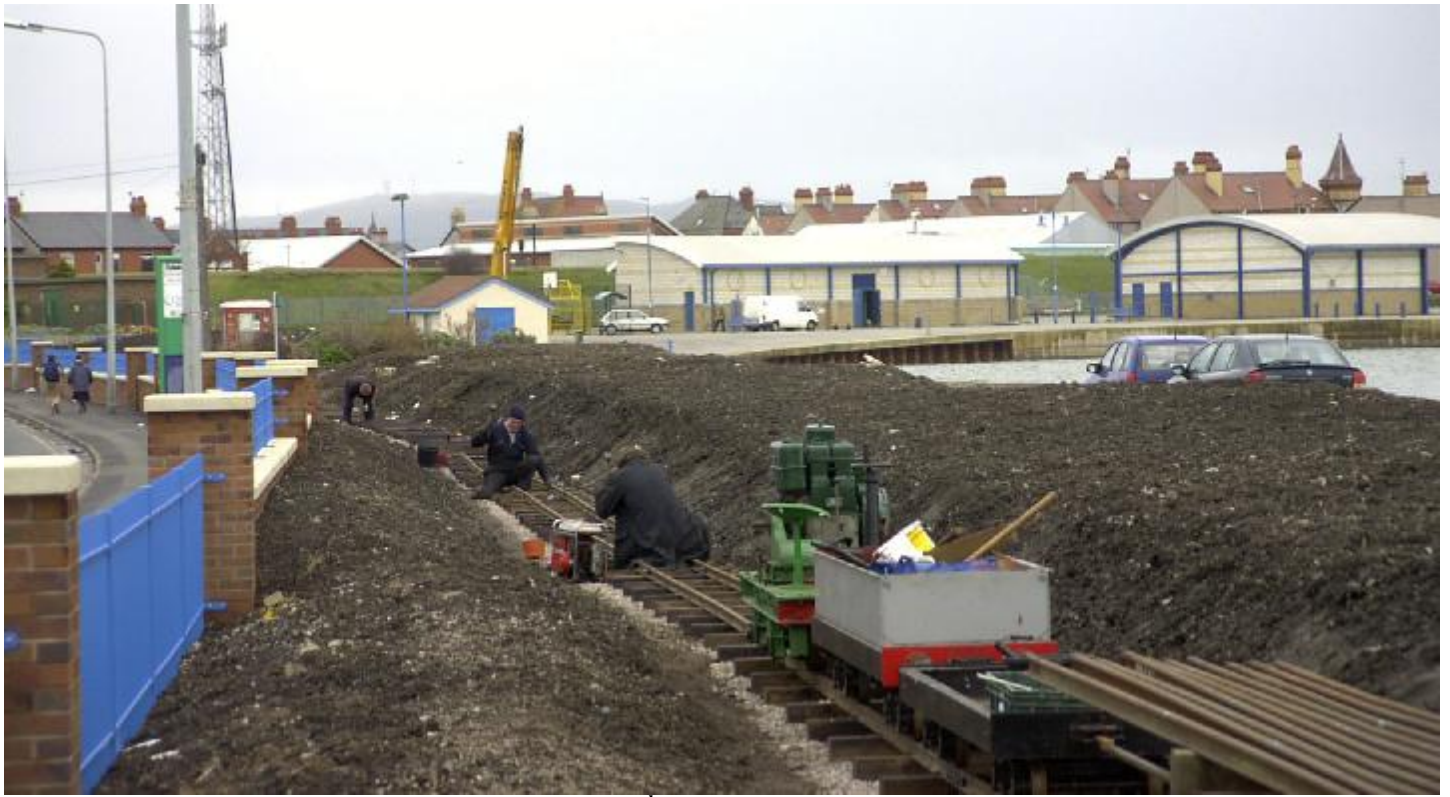
Tracklaying in full swing on Tuesday 4 th March, with our Lister hauled permanent way train.
